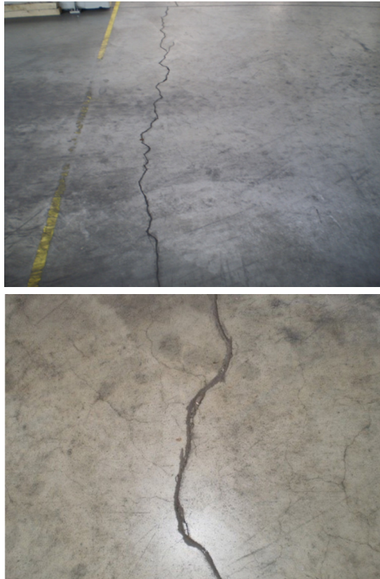
Fig. 2. Cracks of the industrial floor near the entrance to the production hall
