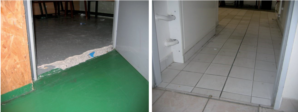
Fig. 4. Threshold failure caused by floor slab lift (left); Visible swelling of the floor with ceramic tiles (right)
