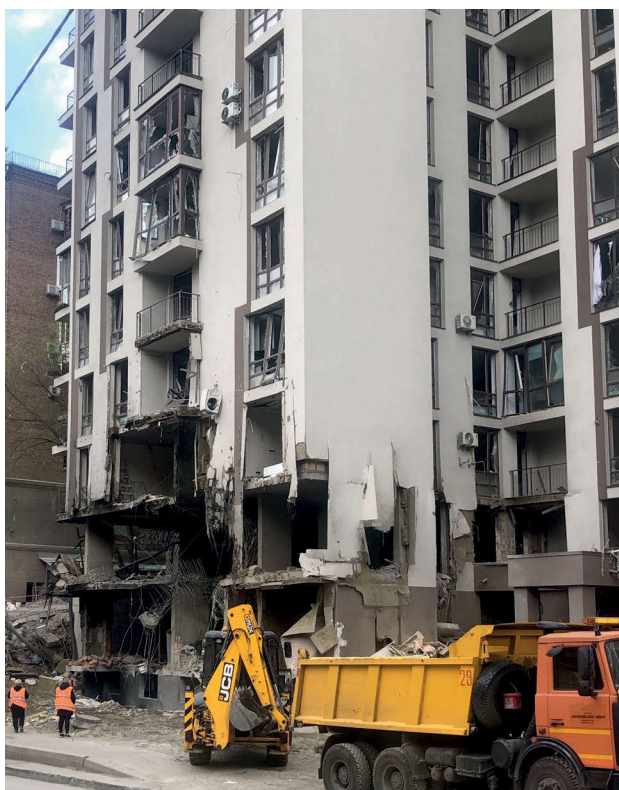
III. 3. Damage to one of the buildings in the 'Lviv Quarter' housing estate. Photo by O. Ivashko.
