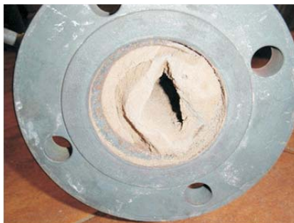
Figure 11. Output of the cyclone to the downcomer pipe.
