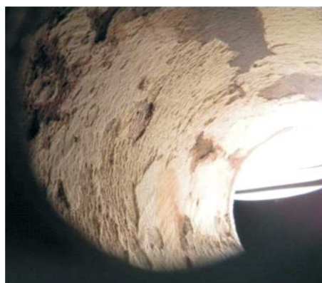
Figure 13. The interior of the position purified of the deposits after the application of EKOSTABIL. The picture was taken in the identical spot where the picture of Fig. 12.
