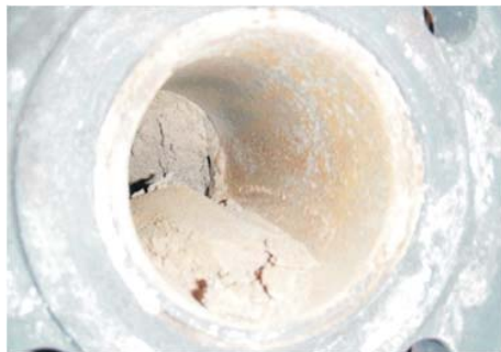
Figure 10. View of junction between the fluidization column and separator.
