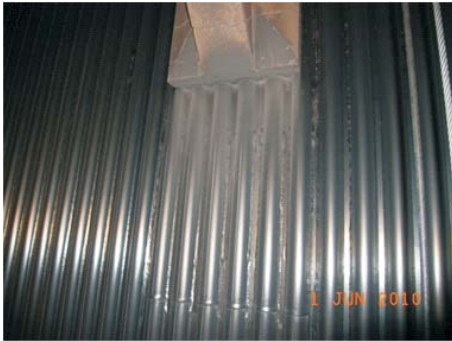
Figure 16. Heating surface, combustion chamber, CFB boiler.
