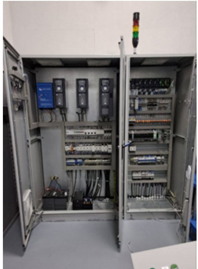
Fig. 6. Control cabinets – drives and automation sections
