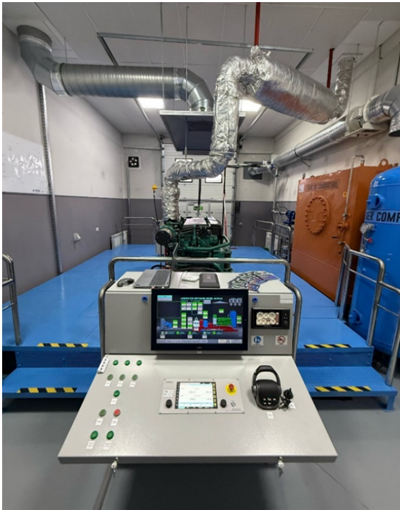
Fig. 7. Control cabinets – drives and automation sections
