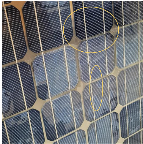
Fig. 2. Delamination of the photovoltaic panel on its surface.
