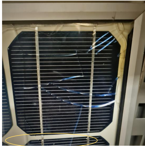
Fig. 4. Front glass breakages as a result of stress.
