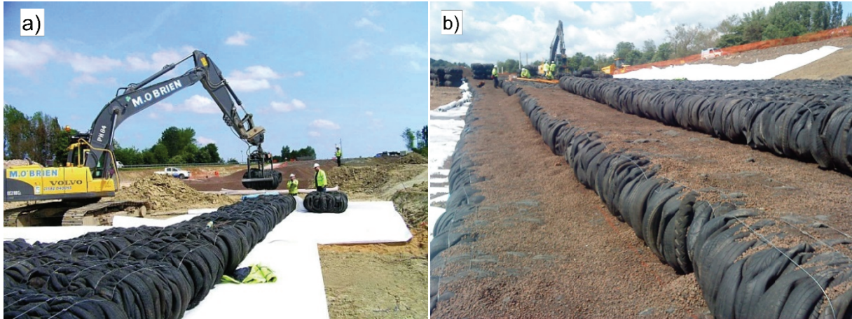
Fig. 2. Construction of lightweight embankment of the A-421 motorway, England: a) tyre bales placed on geotextile; b) tyre bales filled with Maxit [13]
