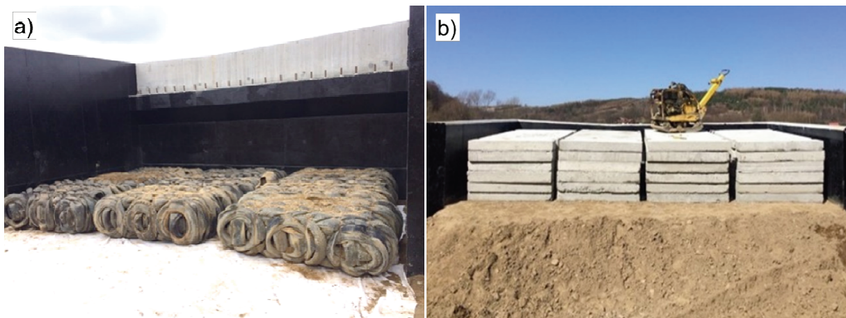
Fig. 10. The abutment backfill of Sielnica bridge, Poland: a) the first layer of tyre bales placed behind the backwall; b) surcharge of tyre bales (A. Duda)
