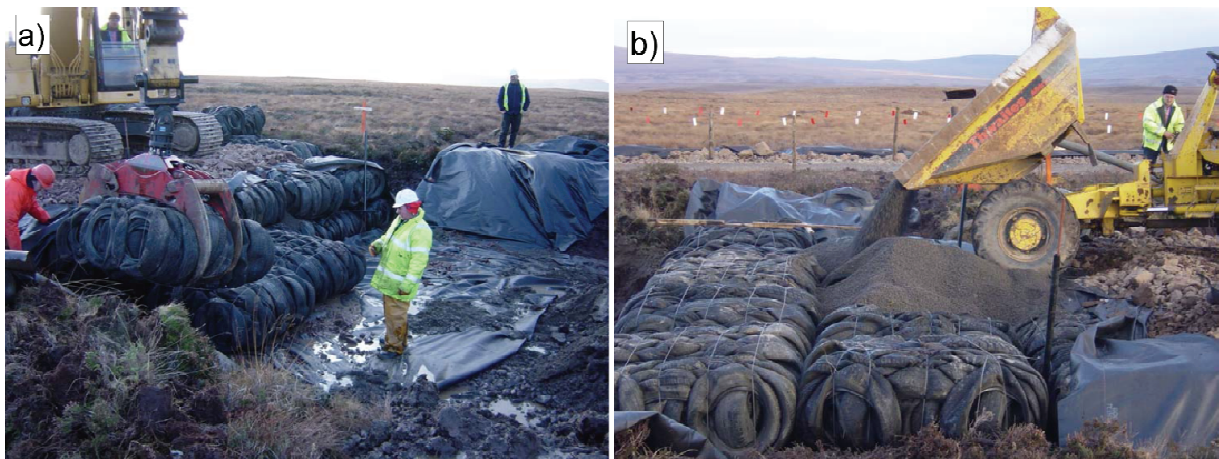
Fig. 5. Tyre bales in the B-871 road foundation, Scotland: a) placing tyre bales on geotextile across the cross-section; b) filling of tyre bales with lightweight aggregate [18]
