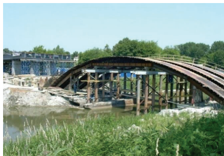
Fig. 3. Concrete arches of the Castle Bridge in Rzeszow: a) general view; b) dense reinforcement of arches; c) steel scaffolding and timber formwork of arches
