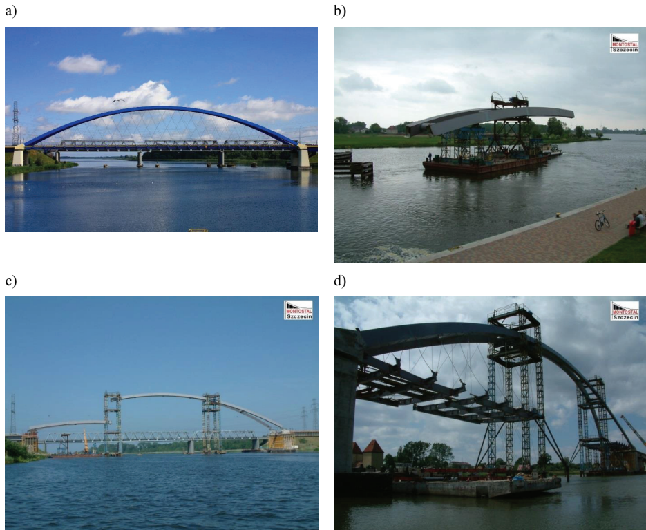
Fig. 24. Steel arch bridge over the Dziwna River in Wolin a) general view; b) Transportation of the part of the arch on the barge c) assembling of the arch d) construction of the deck
