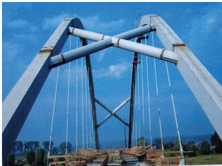
Fig. 19. Bridge over the Warta River along the S3 expressway a) general view; b) erection of arches on steel temporary supports placed on the deck; c) side span assembled on the bank of river
