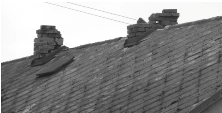
Fig. 6. Characteristic damage of buildings located in the epicentral zone of the M_L = 3.8 mining tremor in Janina mine – cracks and loosening of chimney bricks (V degree of the MSIS intensity)
