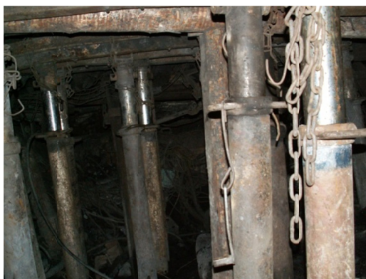
Fig. 1. SHC props supporting a gallery’s roof in the area of the intersection of longwall excavation
