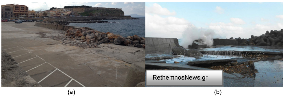
Figure 4 Damages of the base of windward wave breakwater: (a) previous damages, photograph taken on January 4th, 2014; (b) new damages after structural repairs, photograph taken on January 14th, 2015.
